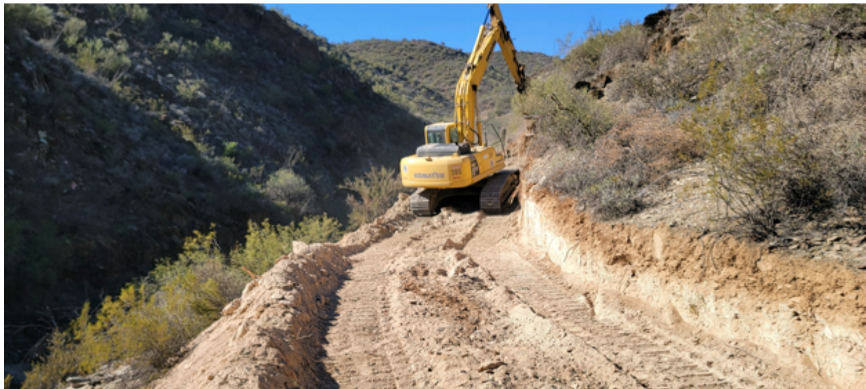
Figure 6. Road construction is underway towards pads W1 and W2 for testing of the Western Target. Drilling from pads W1 and W2 is anticipated to commence in Q1'2023.
